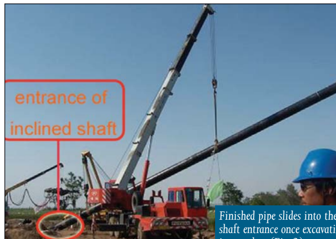
Manual excavation produces inclined slope-traversing pipeline shafts such as the one pictured here (Fig. 1).
